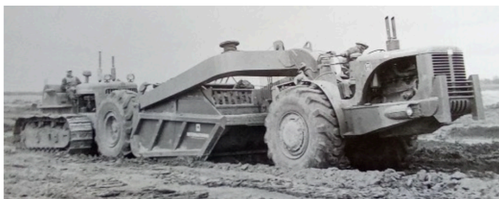
2T-75 scraper and TD-24 crawler working south of Elbow on the canal.
